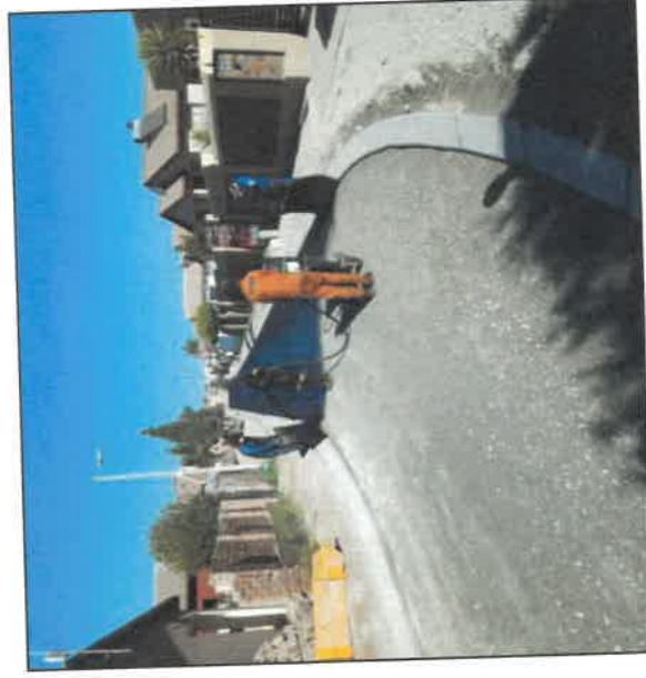
Image 1 & 2: Resurfacing of M2 Highway in Region F and Njambayi Streets in Region D
